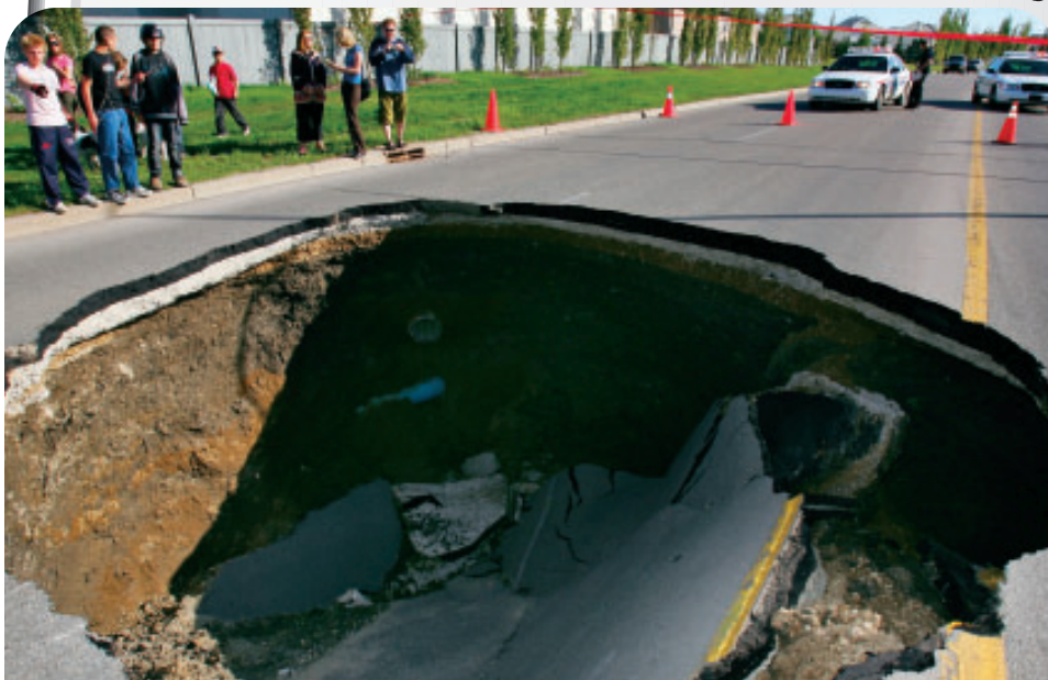
This giant hole appeared on an Edmonton road.
